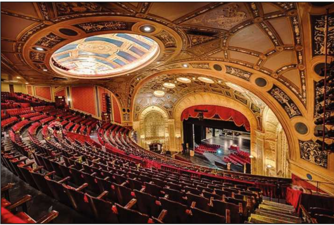
WITH ITS INTERIOR PLASTER and paint ruined by a leaky roof and the elements, and scrapers having taken much of its ornamental hardware, the Capitol Theater in Detroit was a mess in the 1990s when the Michigan Opera Theater decided to make it their new home. A $20 million project led Walbridge-Aldinger using union trades magnificently restored the Detroit Opera House.
